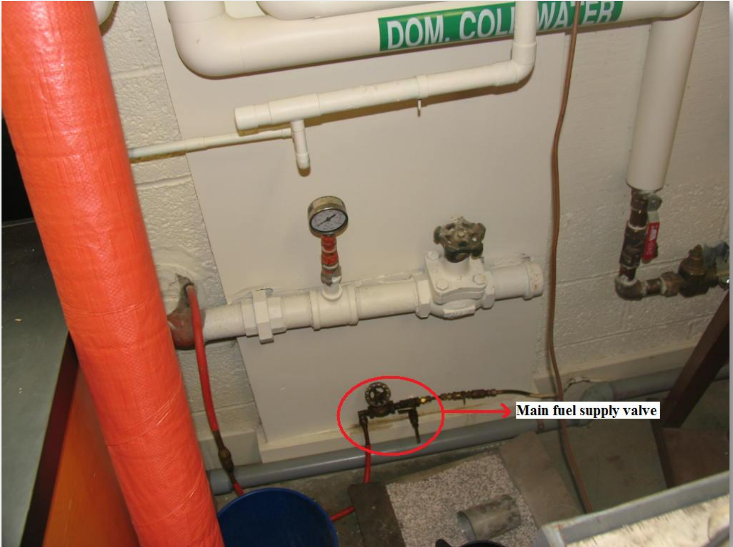
Figure 20: Main fuel supply valve location
