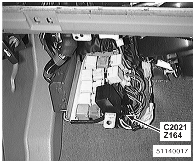
234. behind LH side of fascia (Manual Transmission) Z164 Speed Trip Module C2021 (5-B)
